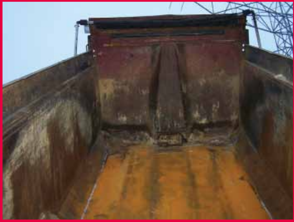
Photograph of a dump box after being in contact with an electrical wire.
