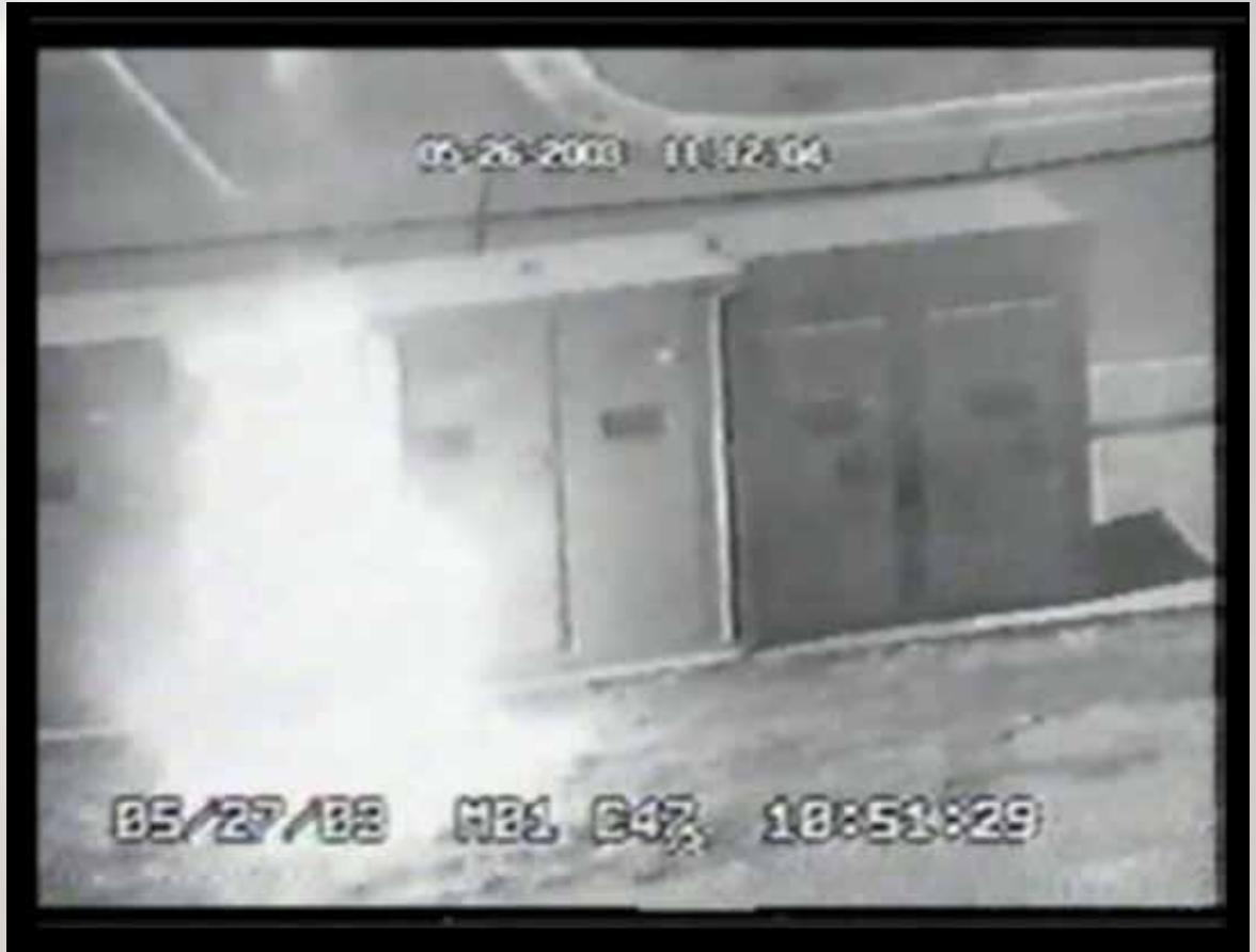
Arc flash can produce a powerful blast and extreme temperatures. The new CSA standard Z462-08 tells companies how to prevent and protect against arc flash in the workplace.
