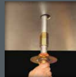
Install V36 Dry Sprinkler with Style AB6 Assembly up through the freezer wall
